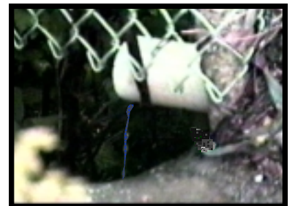
CRAM internal drainage outlet pipe discharging water at Palos Verdes Drive South
