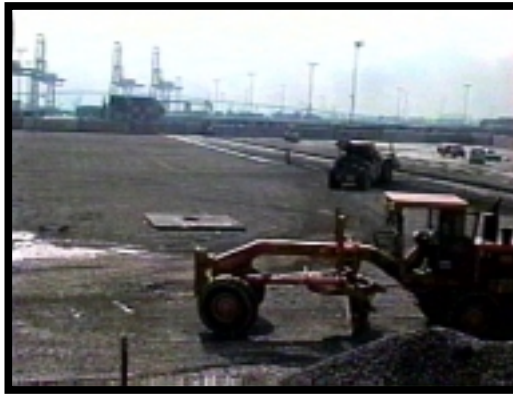
Port of LA CRAM construction site, Jan. 19 continuation of work without further delay
