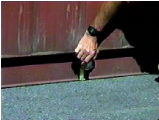
Port of LA CRAM Pavement, typical deformation measurement indicates 1/4" or less rutting in the wheel paths of the top-loader...
