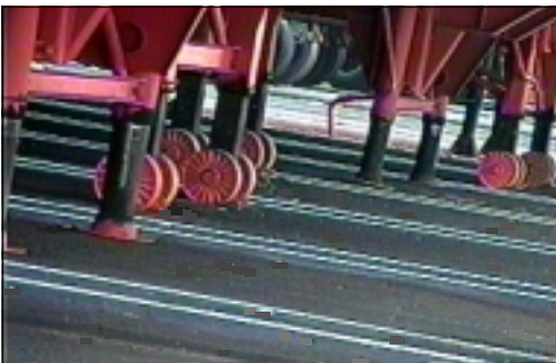
CRAM Pavement; Port of Los Angeles, Berths 127 - 131, supporting loaded chassis landing gear
