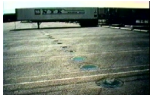
Depressions in the NYK Terminal Conventional Pavement at the Port of Los Angeles caused by loaded chassis landing gear
